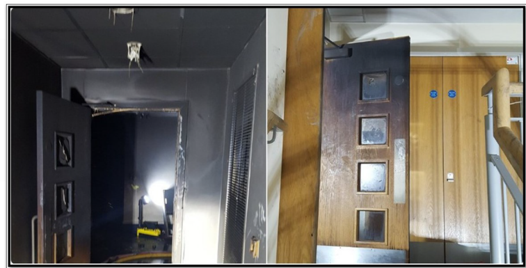
An image of a fire door having done its job
